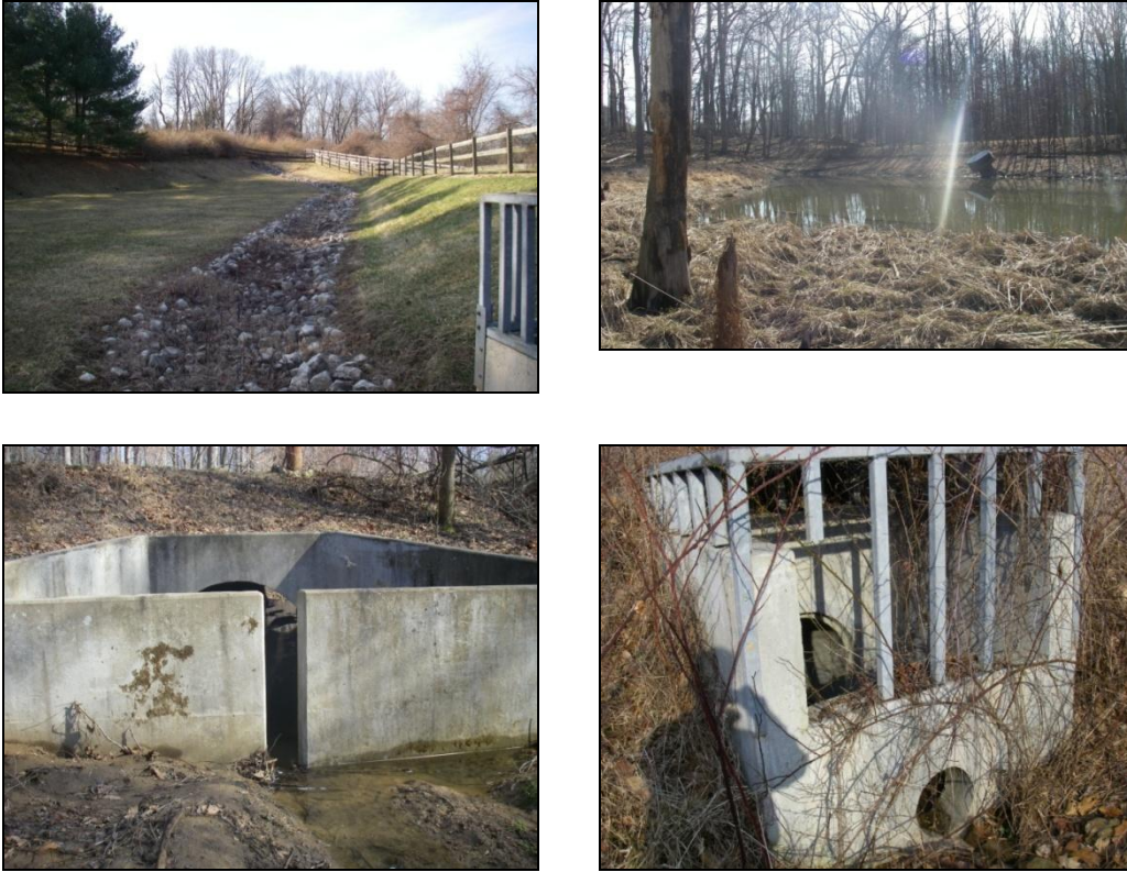
Figure 4-9. Pond #67 riprap channels (top left), Pond #65 leaning riser and trees on embankment (top right), Pond #66 weir wall (bottom left), and Pond # 69 concrete riser structure (bottom right).
