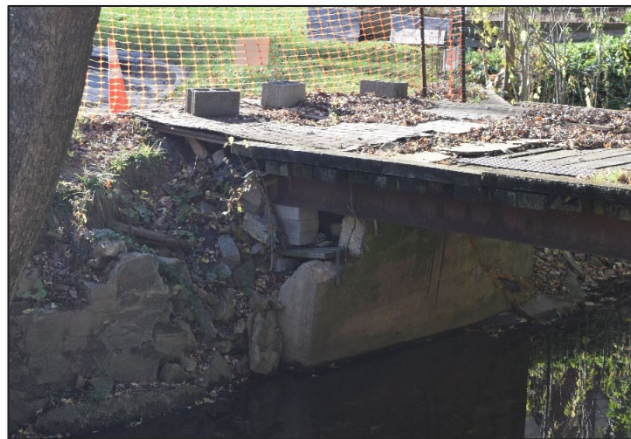
Photograph 9: Bridge 7: Cracked Abutment
