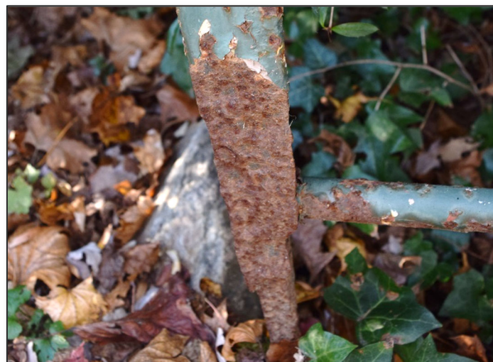
Photograph 6: Bridge 5: Rusted Handrail
